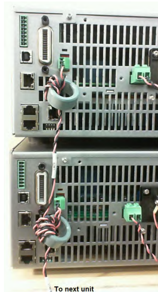
Cables are shown without covers for clarity.
